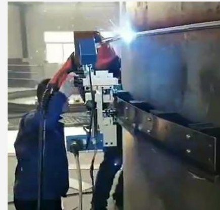
transverse circumferential weld
